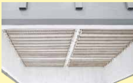
Heating elements in furnace hood
