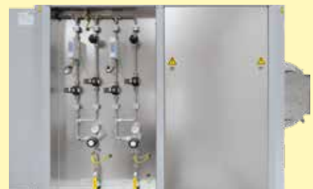
Gas supply system with mass flow controller
