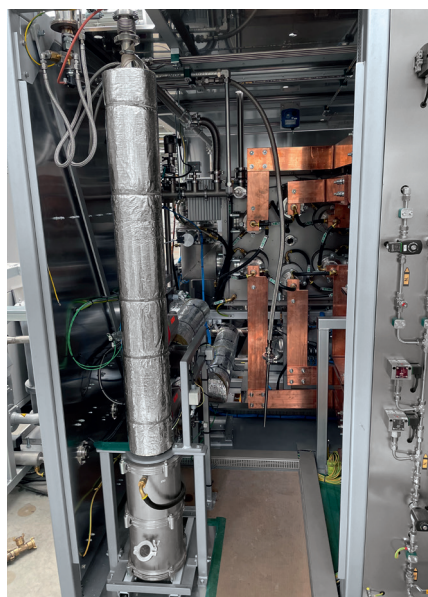
Heated exhaust gas line with binder trap
