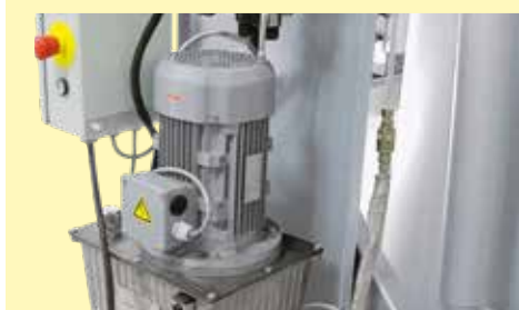
Hydraulic system with flame resistant hydraulic fluid
