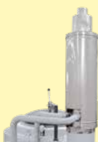
Heat exchanger in the exhaust gas duct
